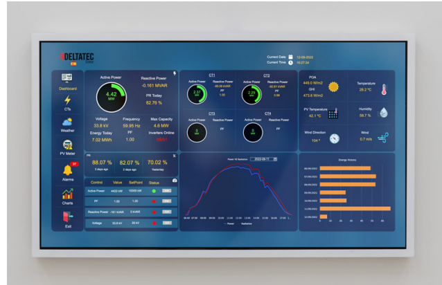
The Kabulasoke PV Plant SCADA System picture.
