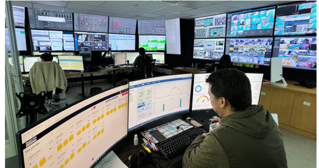
The Chilean Remote Operation Control Center (CROCC) located in "La Serena", Chile
